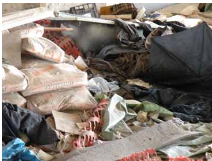
Picture 8.1: A temporary bed of a homeless person addicted to drugs in unfinished buildings in Koper
